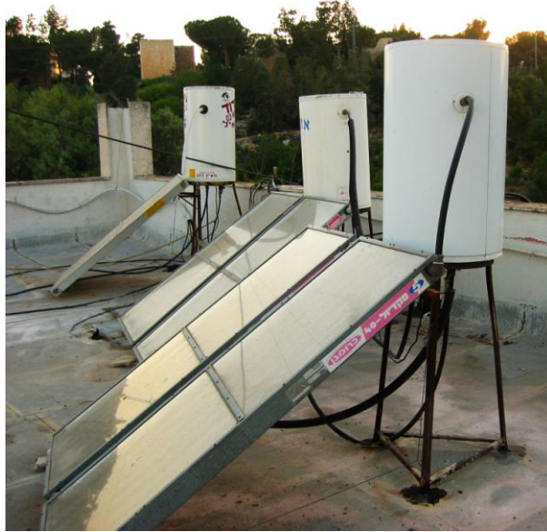
Figure 4. A solar combisystem on the roof of a house used to heat water. (Wikipedia, 2006)
